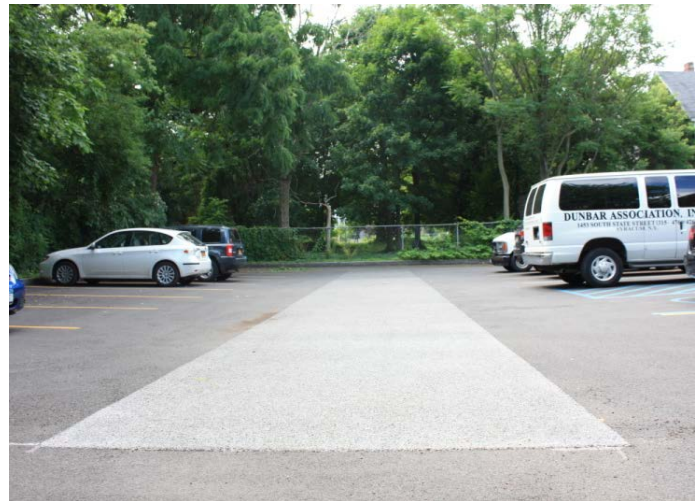
Porous Strip - Parking Lot (view from North)
