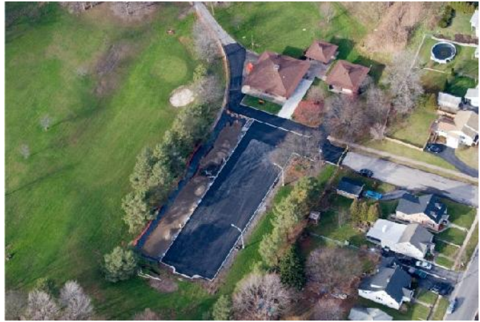
Sunnycrest Golf Course Parking Lot after Pavement Removal & Construction of Bioretention Areas
