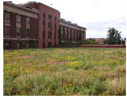
Vegetated Roof at SUNY-ESF in Syracuse, NY
