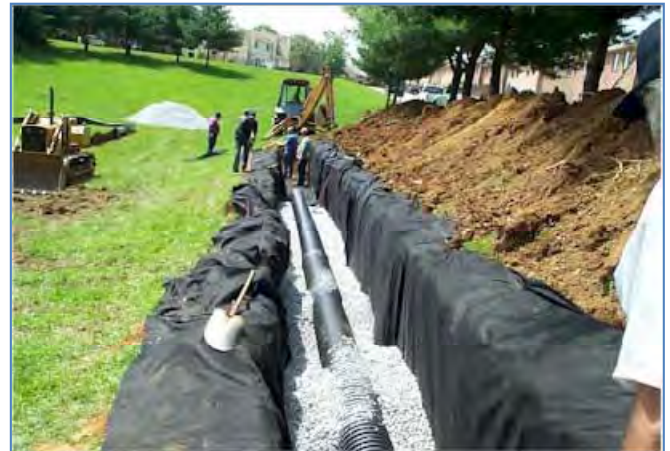
Infiltration Trench in Chester County, PA
