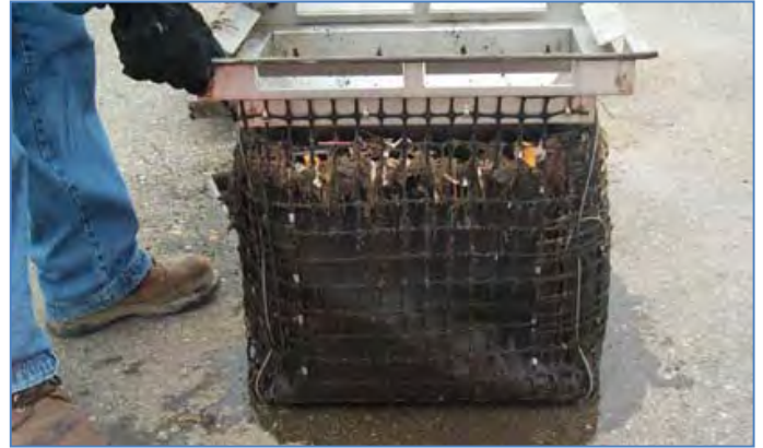
Filtration insert with debris in St. Clair Shores, MI. Source: Environmental Consulting & Technology, Inc
