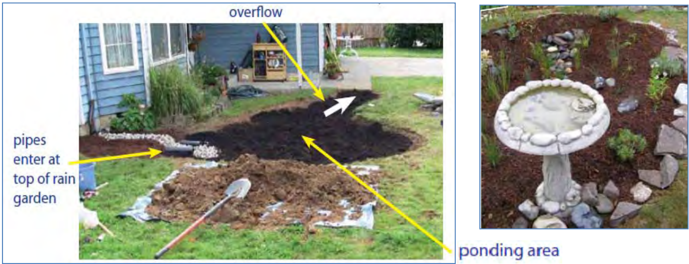
Figure 5: Example of downspout disconnection to rain garden (Source: The City of Gresham, Oregon Website)
