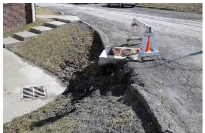
Erosion caused by parking lot runoff at Shove Park before the green infrastructure project was implemented
