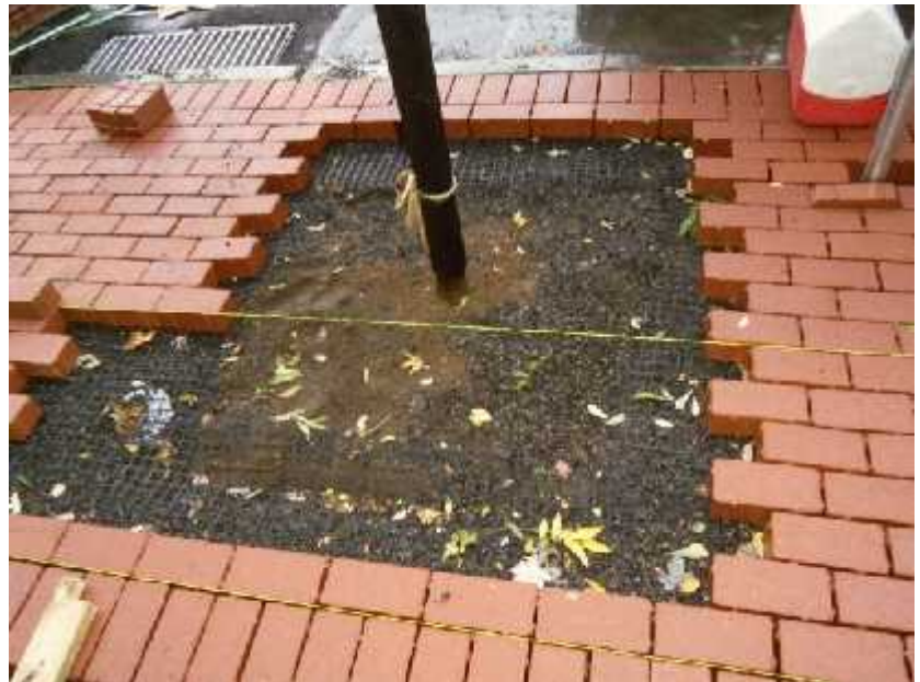
Installation of porous pavers around a street tree on the 200 block of Montgomery Street
