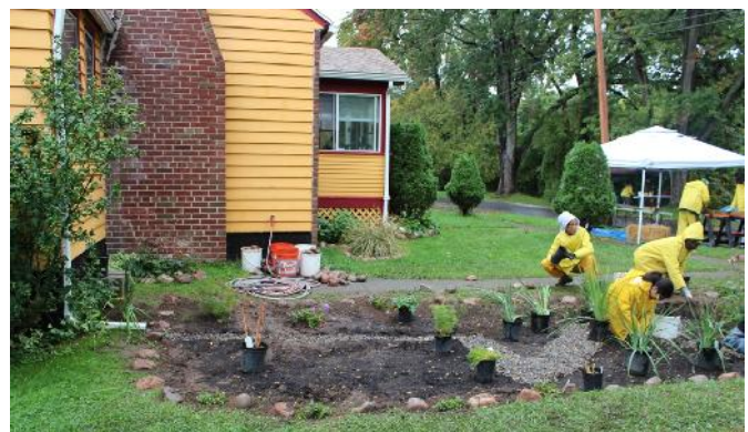
Photos of the Rain Garden Construction by the Onondaga Earth Corps at 133 Vale Street
