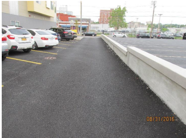
Porous Parking Lot at 712 East Fayette Street
