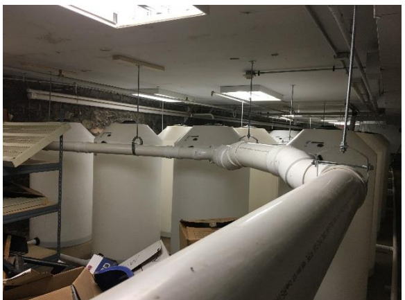
Photos of the installed cisterns
