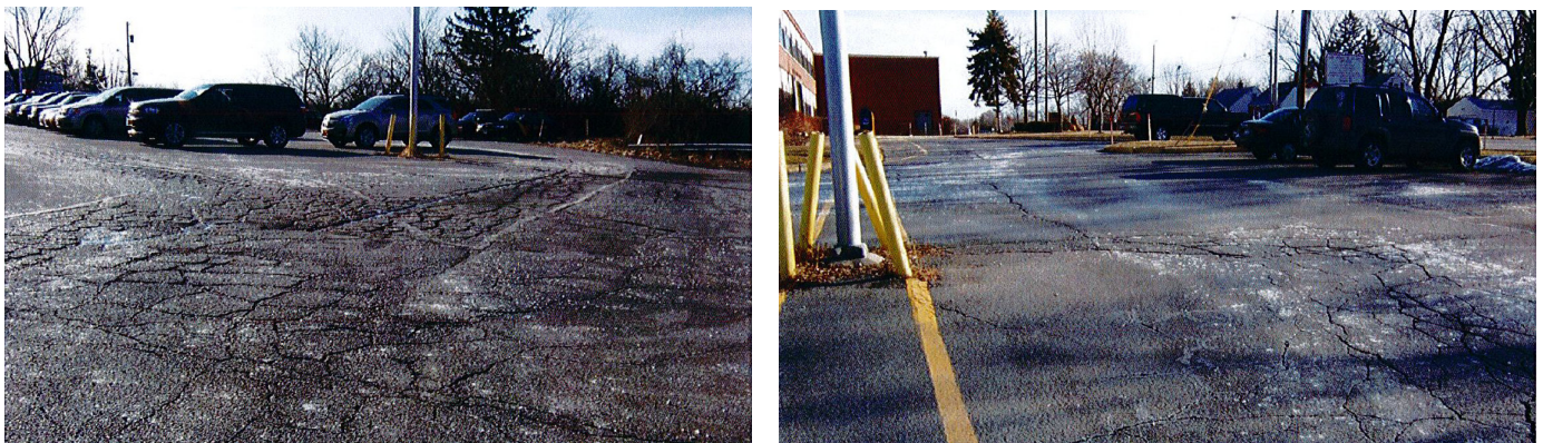
Photos of the Salina Town Hall Parking Lot Prior to Green Infrastructure Installation
