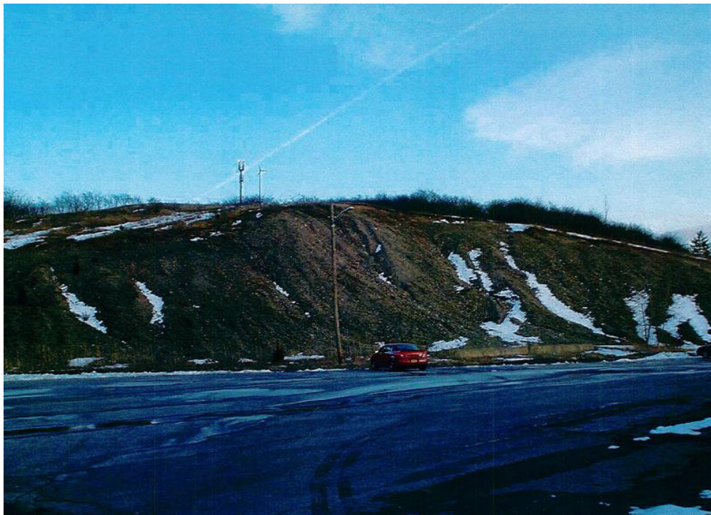
The site of green infrastructure project at Solvay Youth Center. This hill will be stabilized to prevent erosion, and a bioretention system will be installed at the base of the hill.
