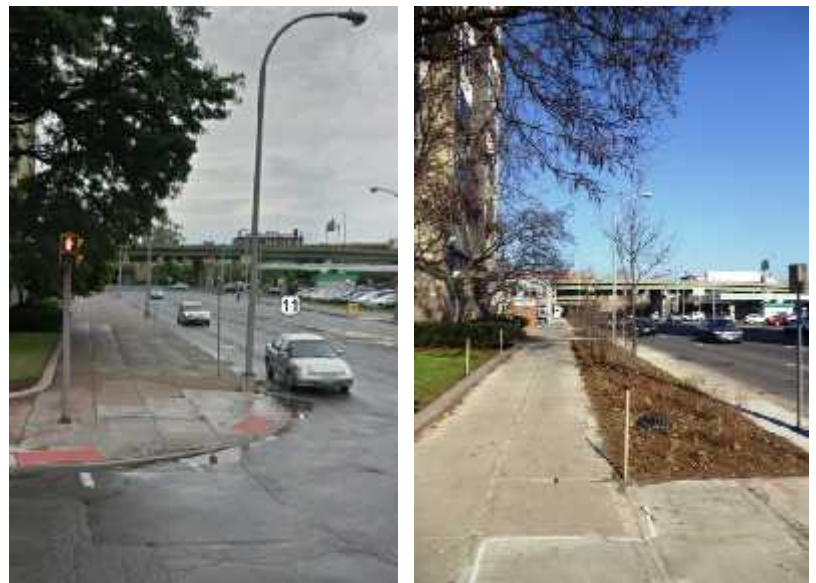
Before and After Installation of Planter Boxes along the 100 Block of S. State Street
