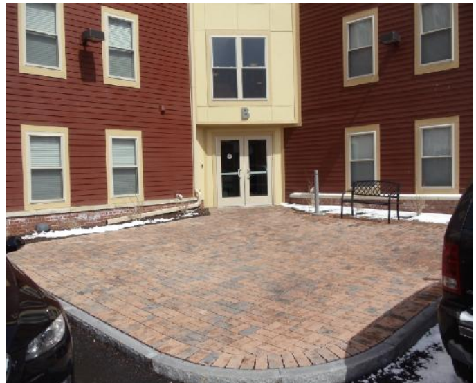
Porous Paver Sidewalk
