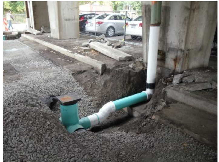
Example of a Disconnected Downspout
