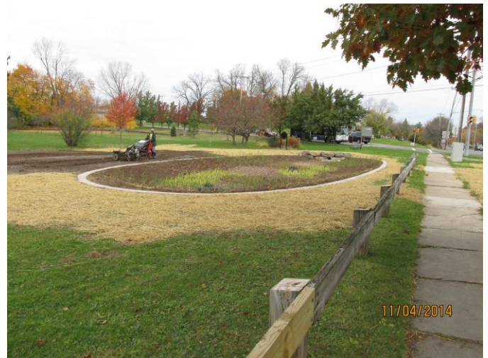
Progress Photo of the Rain Garden Installed at the Northeast End of Comfort Tyler Park
