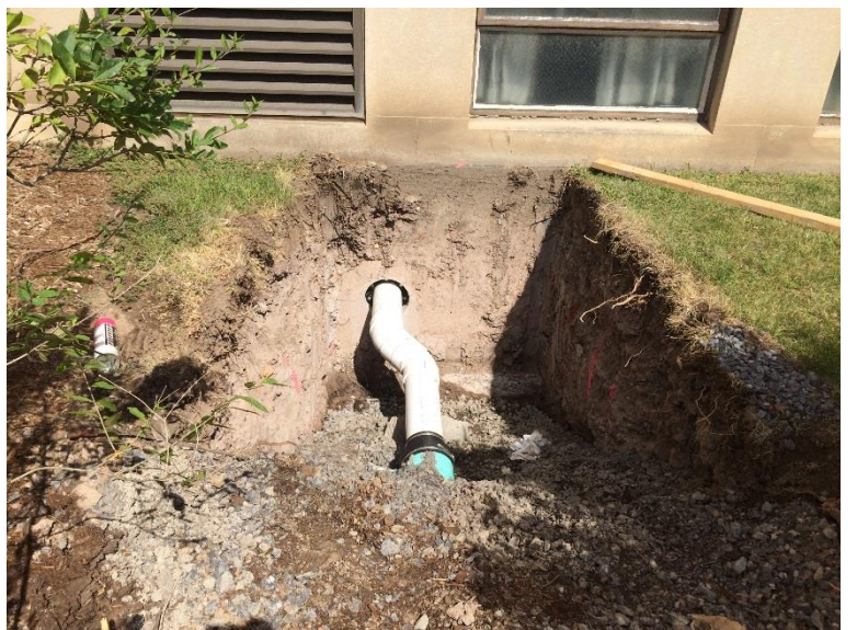
Building Roof Leader Disconnection and Plumbing to the Green Infrastructure System
