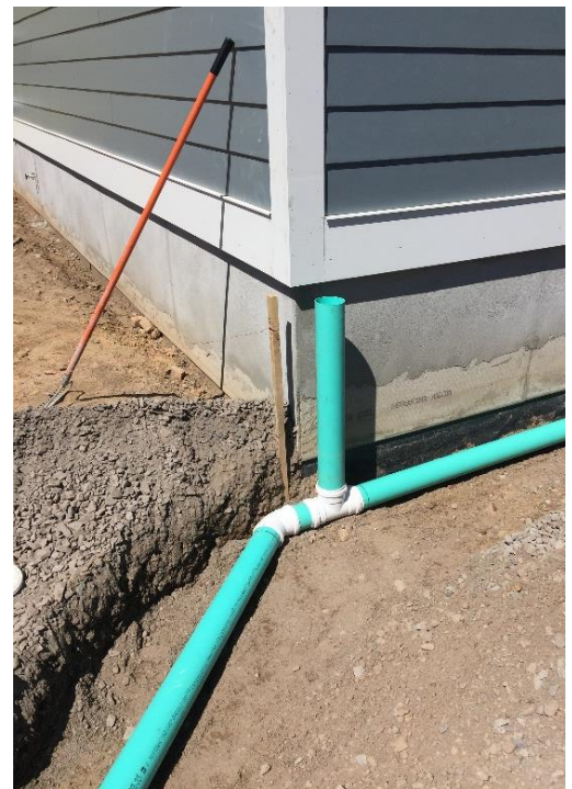
Roof Leader Disconnection to the Underground Infiltration Basin
