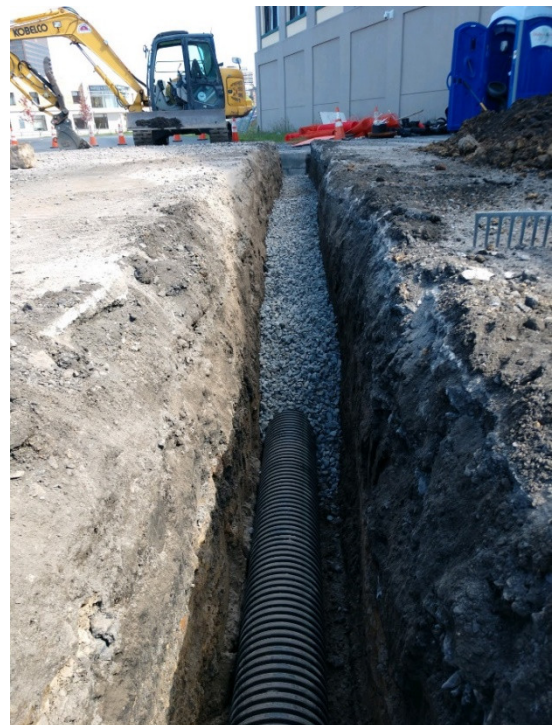
Disconnection of the roof drain from the adjacent building and plumbing to the installed green infrastructure
