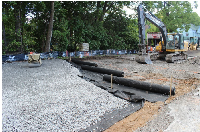
View of parking lot under construction, laying of geotextile and stone before porous pavement is laid
