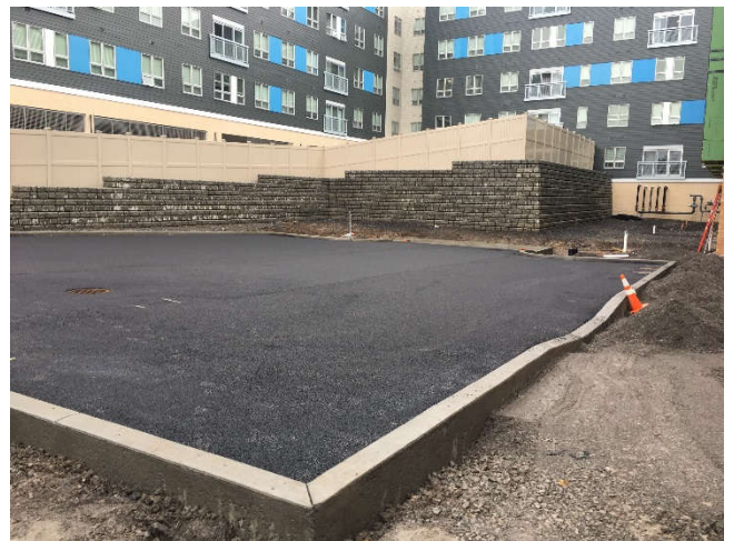
Porous Asphalt Parking Lot, Added Green Space Areas Around Perimeter of the Lot in Progress
