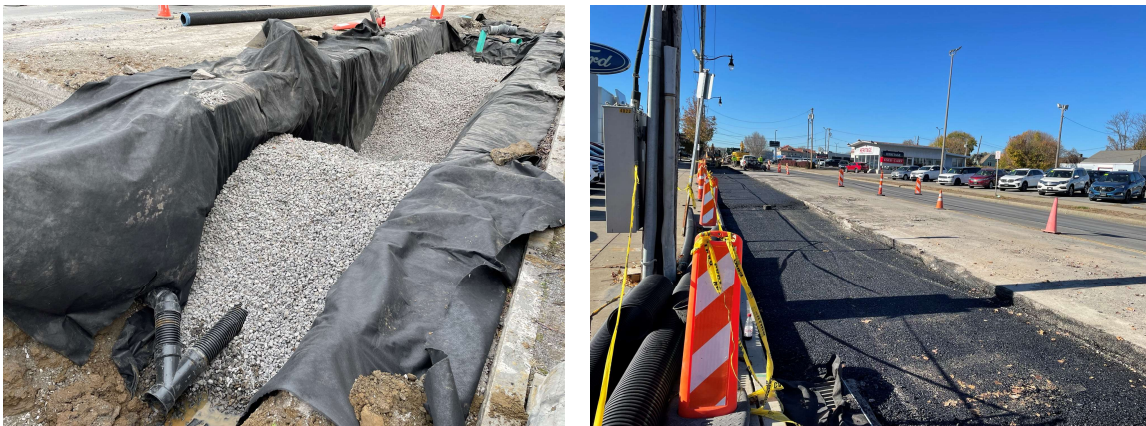
Construction of the West Genesee Street Green Street project in CSO 066 was completed in 2022
