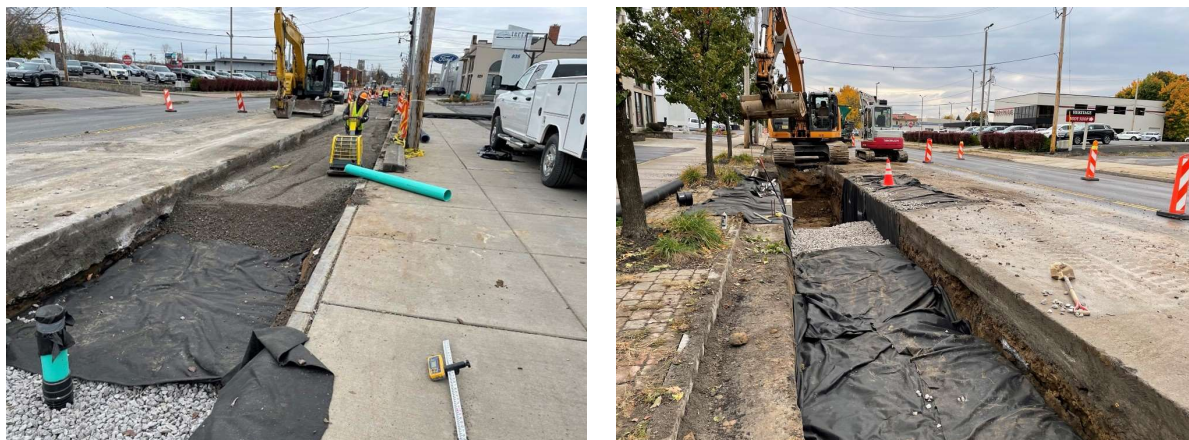
Construction photos of the West Genesee Street Green Street Project. Several underground infiltration trenches were installed along the project length.
