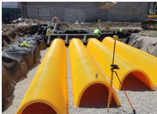
Construction of the underground detention basins at the JMA Parking Lot (GIF #180)
