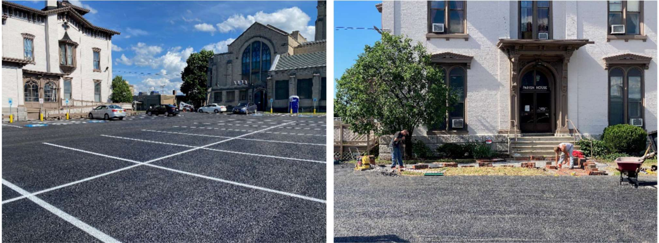
Photographs of the Missio Church GIF project porous pavement parking lot (left) and added green space with GIF pavers (right) being installed.
