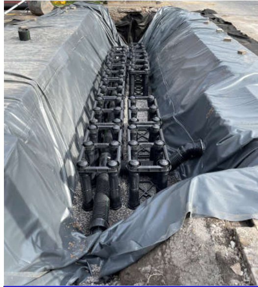
Construction of the Butternut Street Green Corridor project was completed in 2023. The project is in CSO 020 and consists of infiltration trenches, street trees, bioretention, and porous pavers that are estimated to capture 4.2 MG of runoff on an annual basis once complete.
