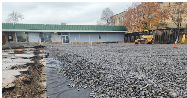
Construction of the Evergreen Manufacturing GIF project in CSO 039 was completed in 2024 and featured a porous asphalt parking lot
