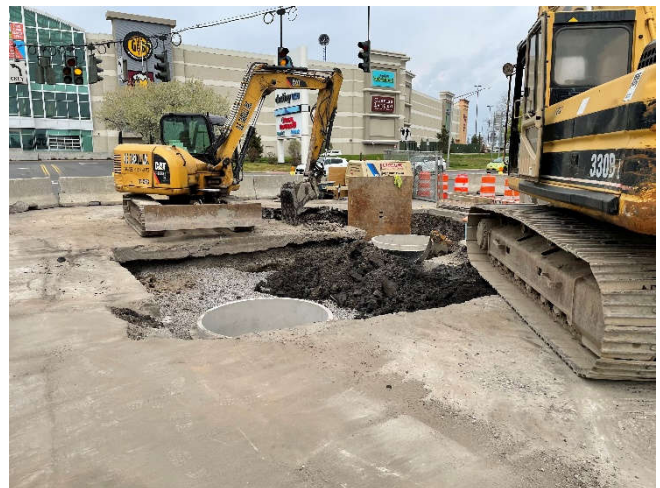
Photo showing the two new manholes in the intersection of Solar St and Hiawatha Blvd
