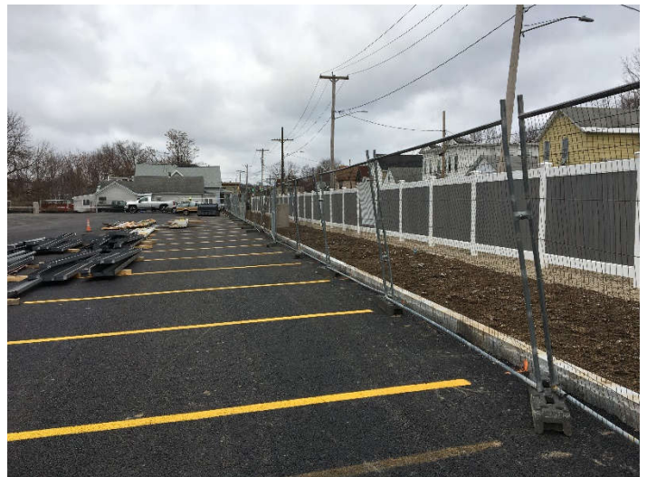
Completed driveway for the Ranalli ALA project. Next spring, the soil strip to the right will be grown in
