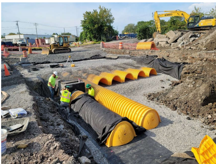
Installation of the capture and slow release chamber system
