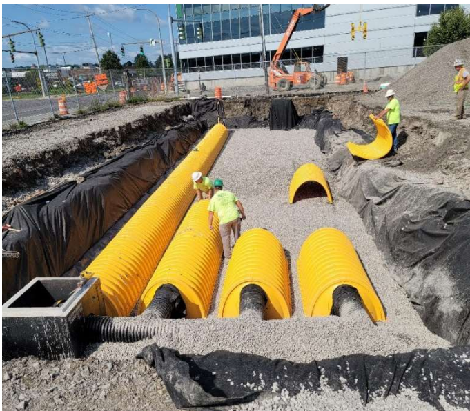
Installation of capture and slow-release chamber system
