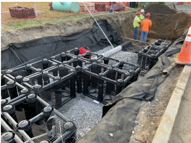
Photo of Silva Cell Installation to Provide Subsurface Soil Volume for Robust Urban Tree Growth
